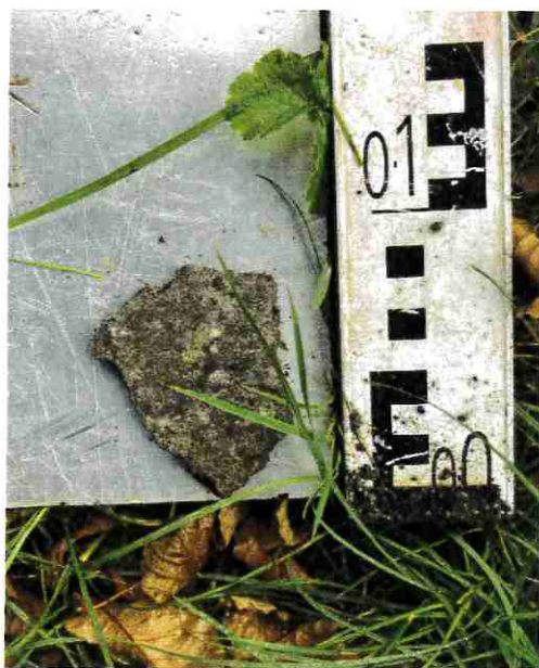
Figure 1, Confirmed Asbestos Cement fragment.
